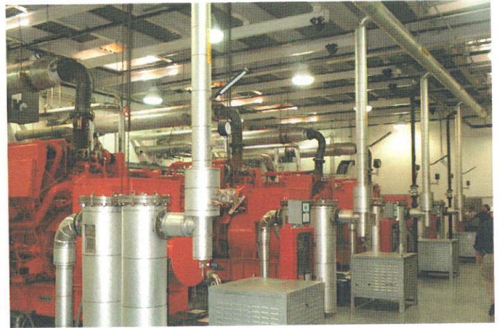
Chapter members visit the landfill generator station and view the four Waukesha engines (One is slated for future use upon an increase in gas flow.)
