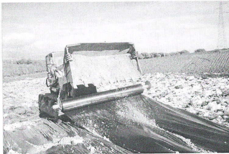
Here the Enviro Cover plastic film is placed by the Enviro Cover Deployer attached to the bucket of a loader
